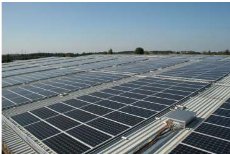
Solar panels (source: Flickr cc)
